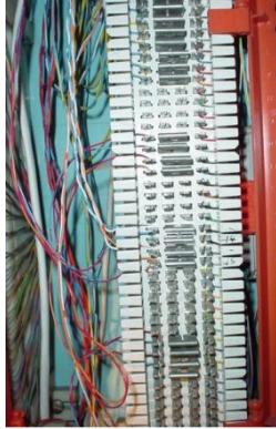
TELEPHONE SYSTEM PUNCH-DOWN BLOCK
